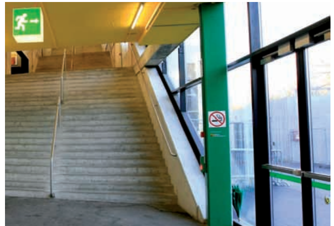
^ Escape doors in heavily frequented areas require regular maintenance to ensure that they can operate without problems for many years.
